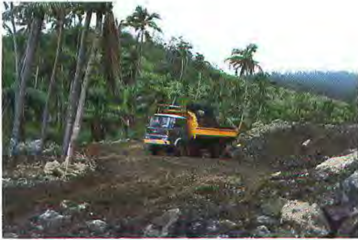
Fig. 13 Cutting a road through a tropical rain forest. The road not only destroys the natural vegetation, it also opens up the forest to further exploitation.
